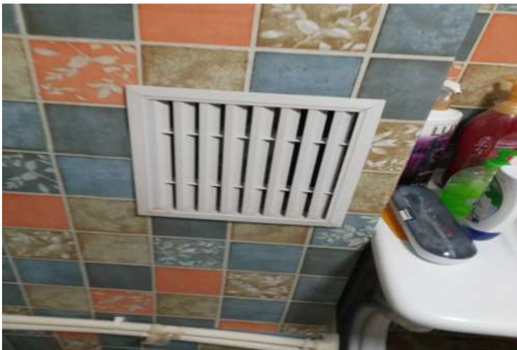
Figure 4 Bathroom vent carrying offensive odors from other apartments.
