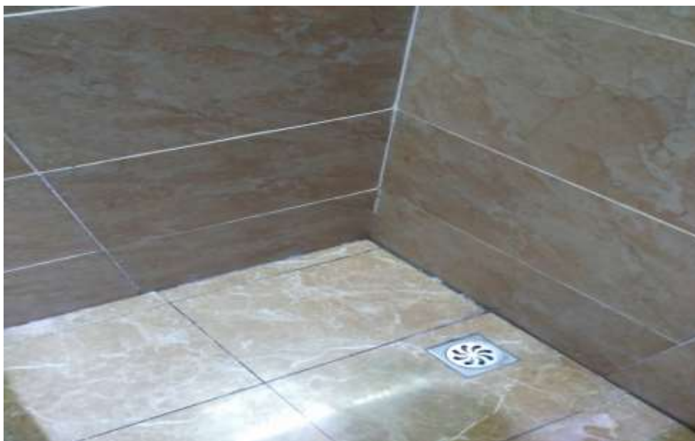
Figure 2 Typical Chinese shower floor with a drain, which doesn't have a trap.
