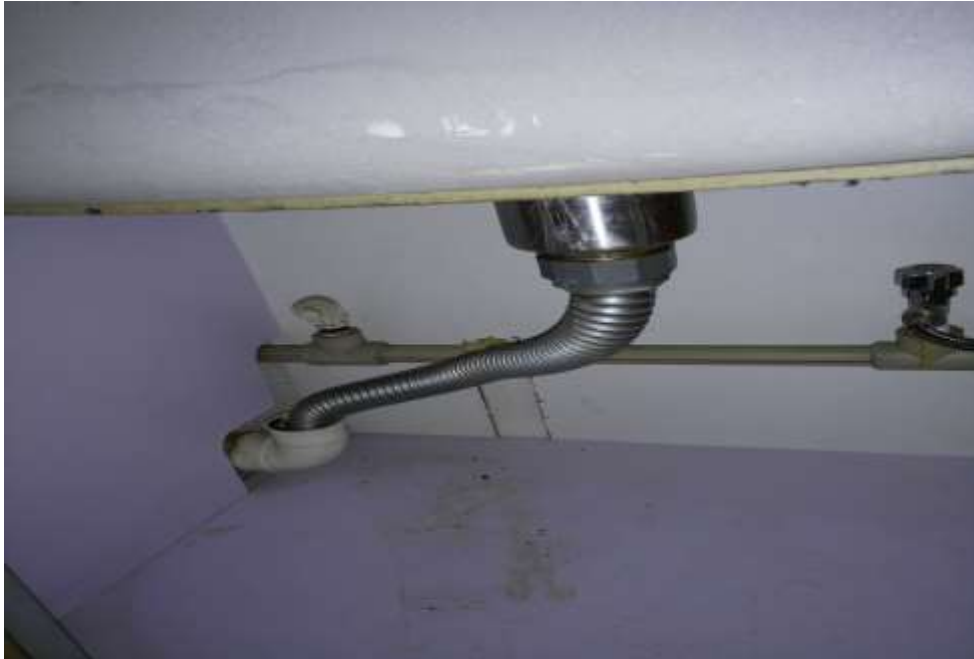
Figure 3 Flexible pipe connection in the kitchen without the water trap showing exposed unsealed drain pipe.
