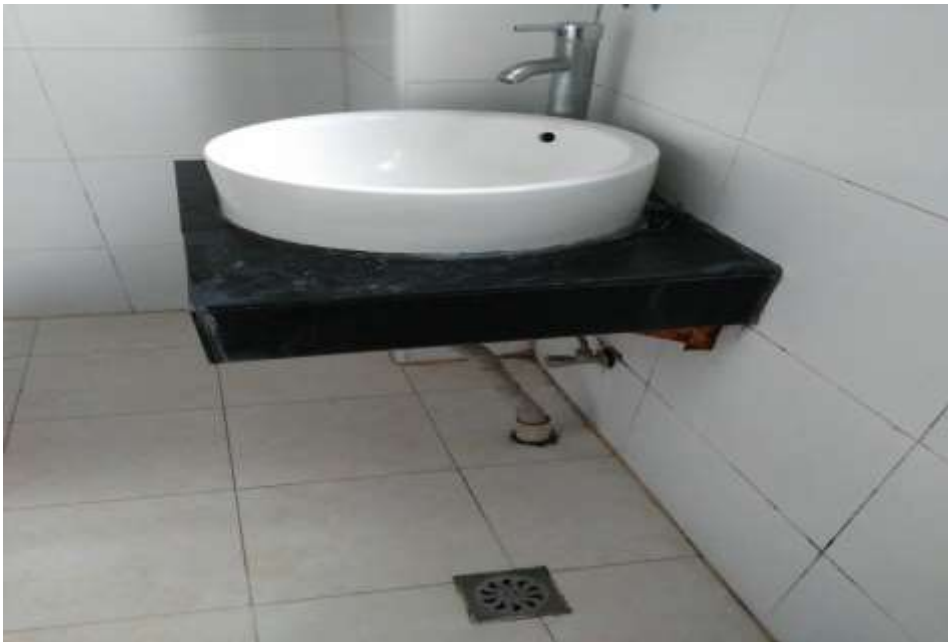
Figure 1 Photo of a typical Chinese bathroom showing a sink without water trap, unsealed sewage line and floor drain without a trap.
