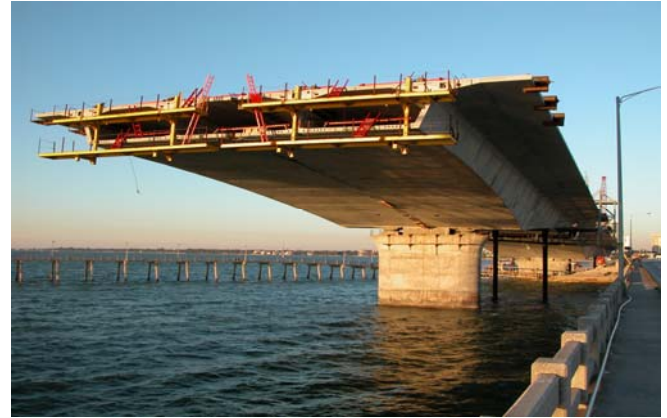
Ringling Causeway Bridge Pier founded on two, 9ft diameter drilled shafts (Sarasota, FL).
