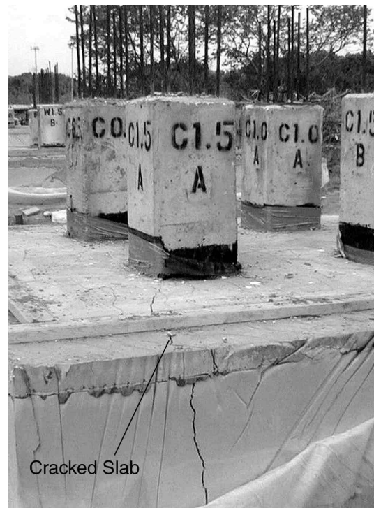
Fig. 16—Seal slab cracks during testing.
