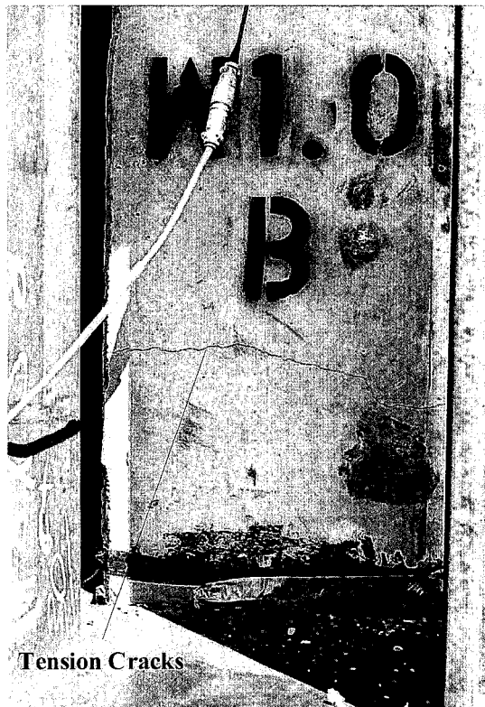
Figure 15: Pile Cracks During Loading
