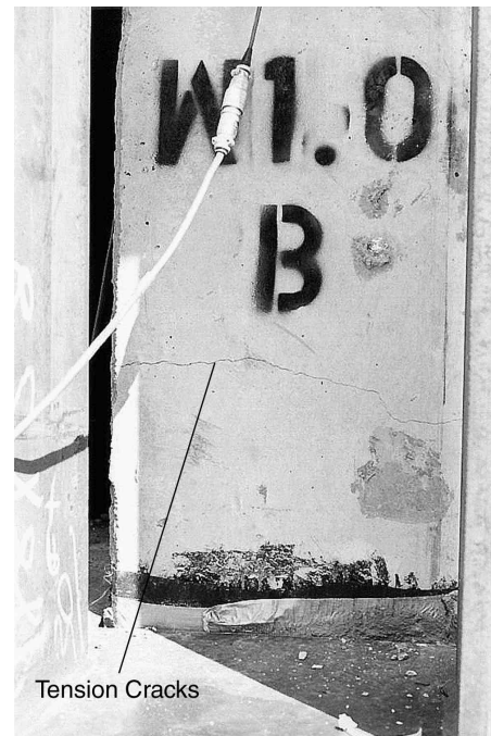
Fig. 15—Pile cracks during loading.
