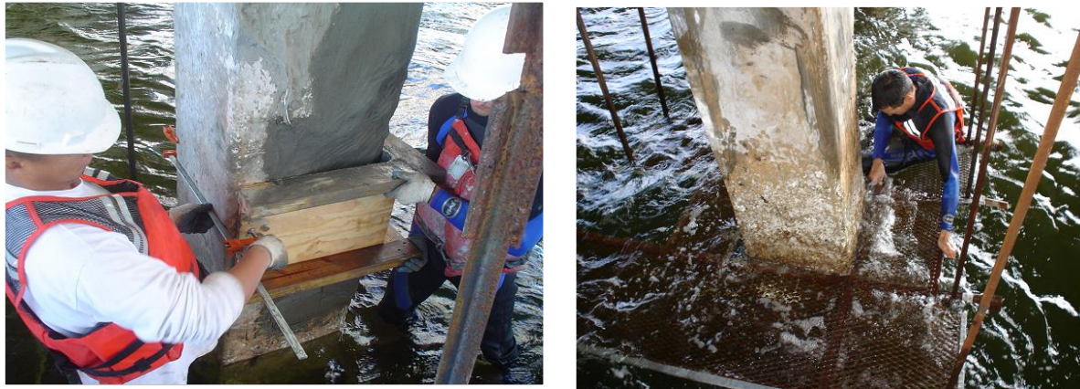
Figure 2. Patching damage (left) and grinding surface (right).
