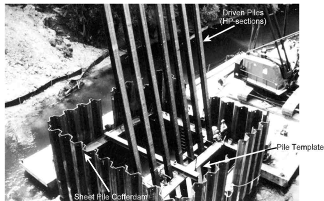
Fig. 1—Sheet pile cofferdam with pile-driving template. (Photo courtesy of Applied Foundation Testing.)
