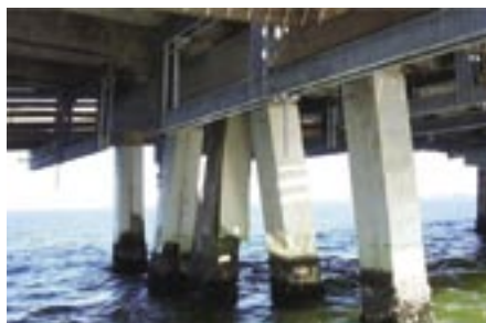
Fig. 1: Piles of the Friendship Trail Bridge that have been previously repaired using concrete jackets
