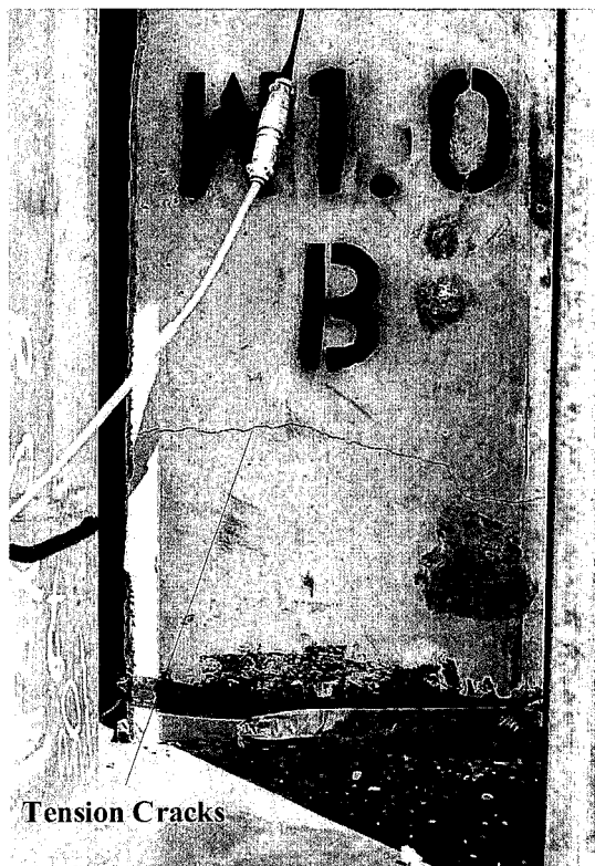
Figure 15: Pile Cracks During Loading
