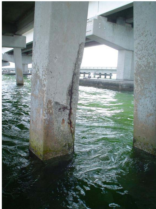
Figure 8 -- Heavily Corroded Pile, Gandy Bridge, Tampa
