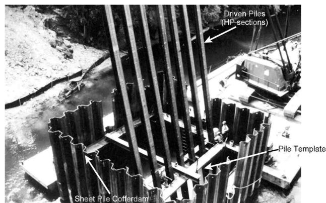
Fig. 1—Sheet pile cofferdam with pile-driving template. (Photo courtesy of Applied Foundation Testing.)
