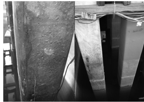
Fig. 5—Surface cracks on unwrapped specimens.
