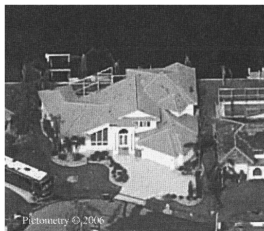
Fig. 7. Home with minor damage. 0.46–9.29 m 2 (5–100 ft 2 ) of missing tiles (Reprinted with permission, Pictometry International Corp. 2006).
