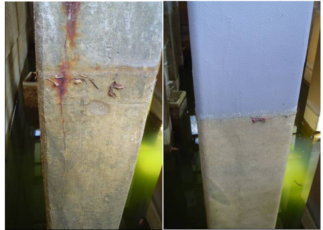
Fig. 5 Cracked control (L) vs uncracked FRP wrapped specimen (R)
