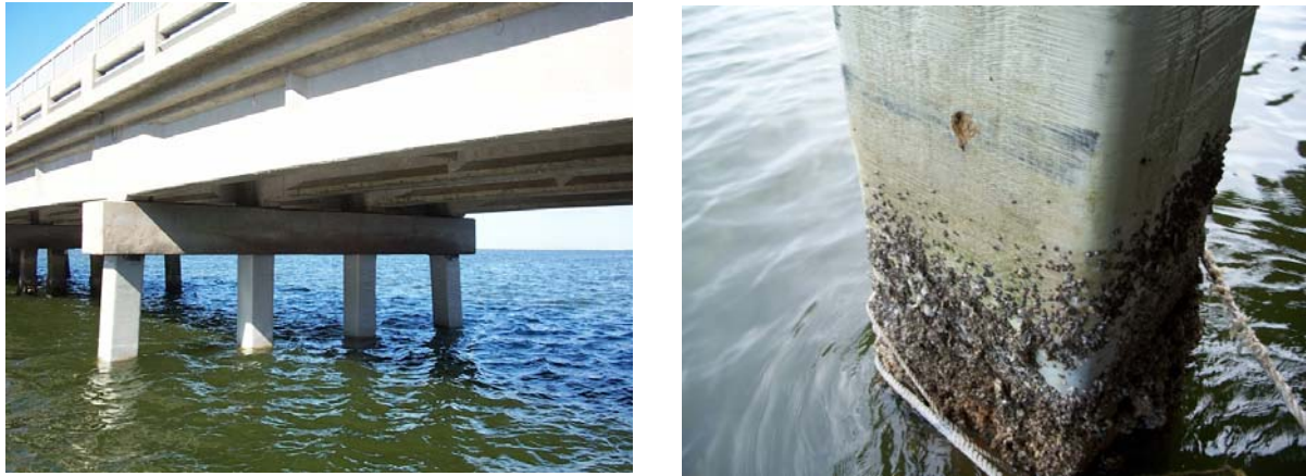
Figure 4. View of FRP wrapped piles when new (left) and after 2 years (right)
