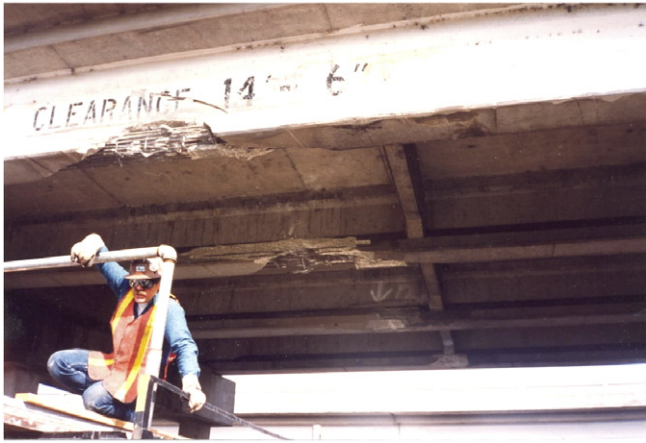
Fig. 1. Damage to prestressed girder due to vehicular collision (Courtesy A. Alvi).
