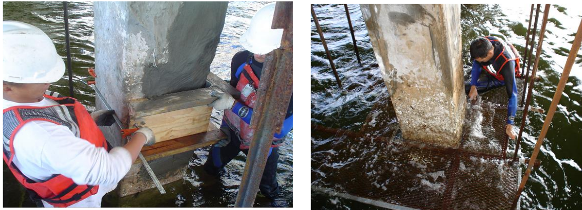
Figure 2. Patching damage (left) and grinding surface (right).
