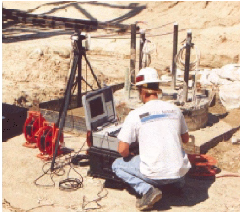
Figure 19 Cross-hole sonic logging of 4 ft diameter shaft (Courtesy of Applied Foundation Testing, Inc.).
