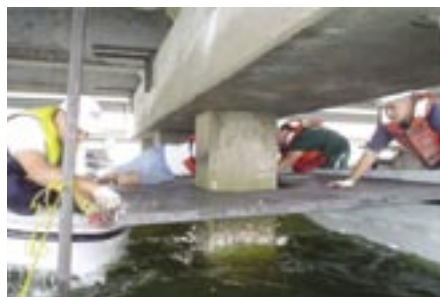
Fig. 4: Installation of scaffold around the four piles in Bent 100. Wood railing was subsequently bolted to the steel angles to delineate the extent of the underwater platform
