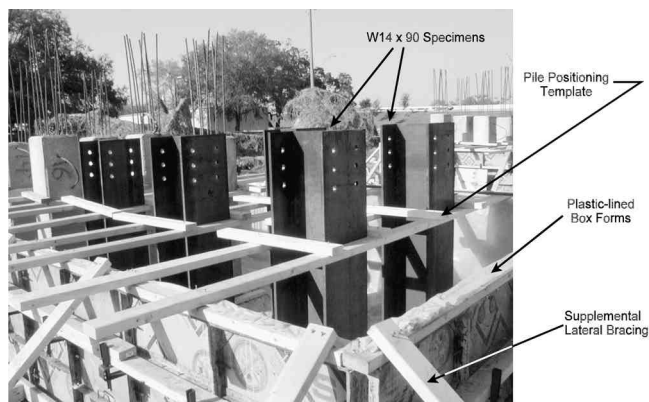
Fig. 5—Steel piles in simulated cofferdam. (Prestressed piles were also tested in the same bed.)
