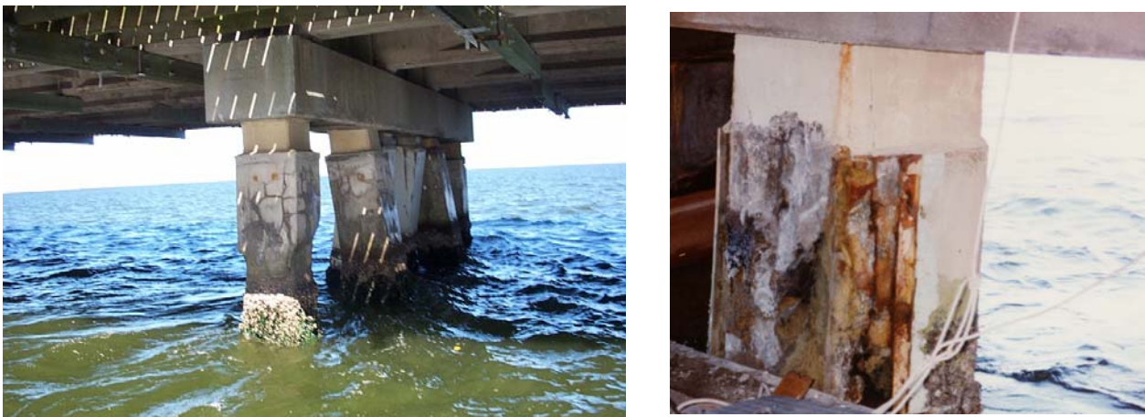
Fig. 1. View of jacketed piles (left) and view of underlying corrosion with the jacket removed (right)
