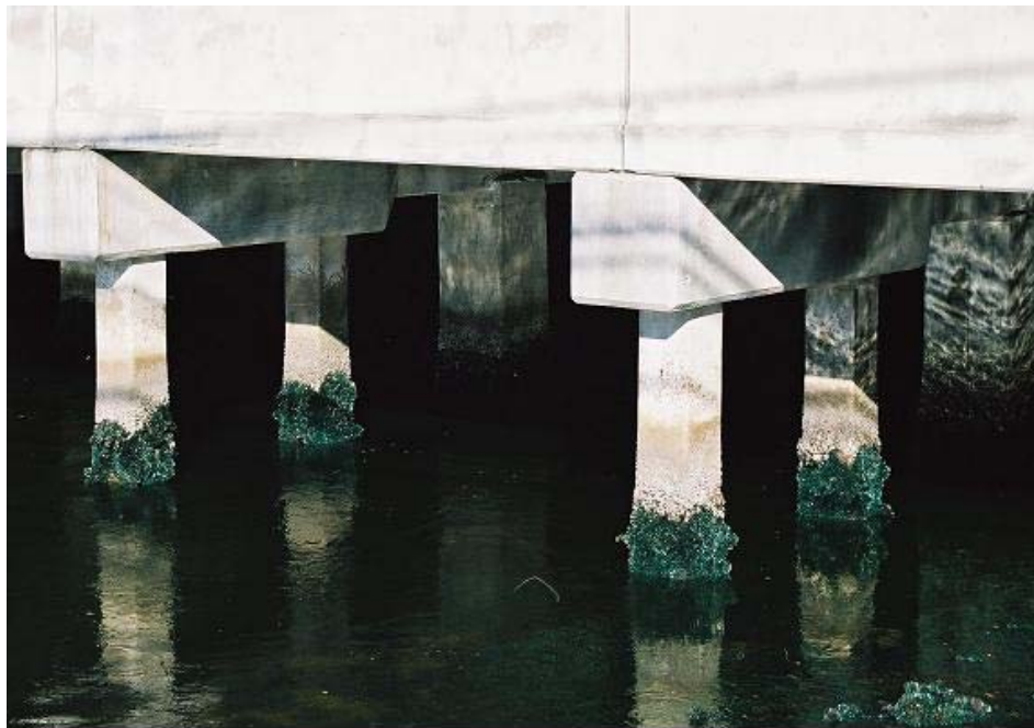
Figure 2 -- Marine Growth, Allen Creek Bridge, Clearwater
