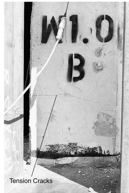
Fig. 15—Pile cracks during loading.
