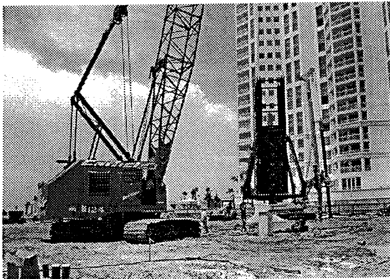
Figure 2.10 Entire mechanism can be placed on the next test pile without disassembly.
