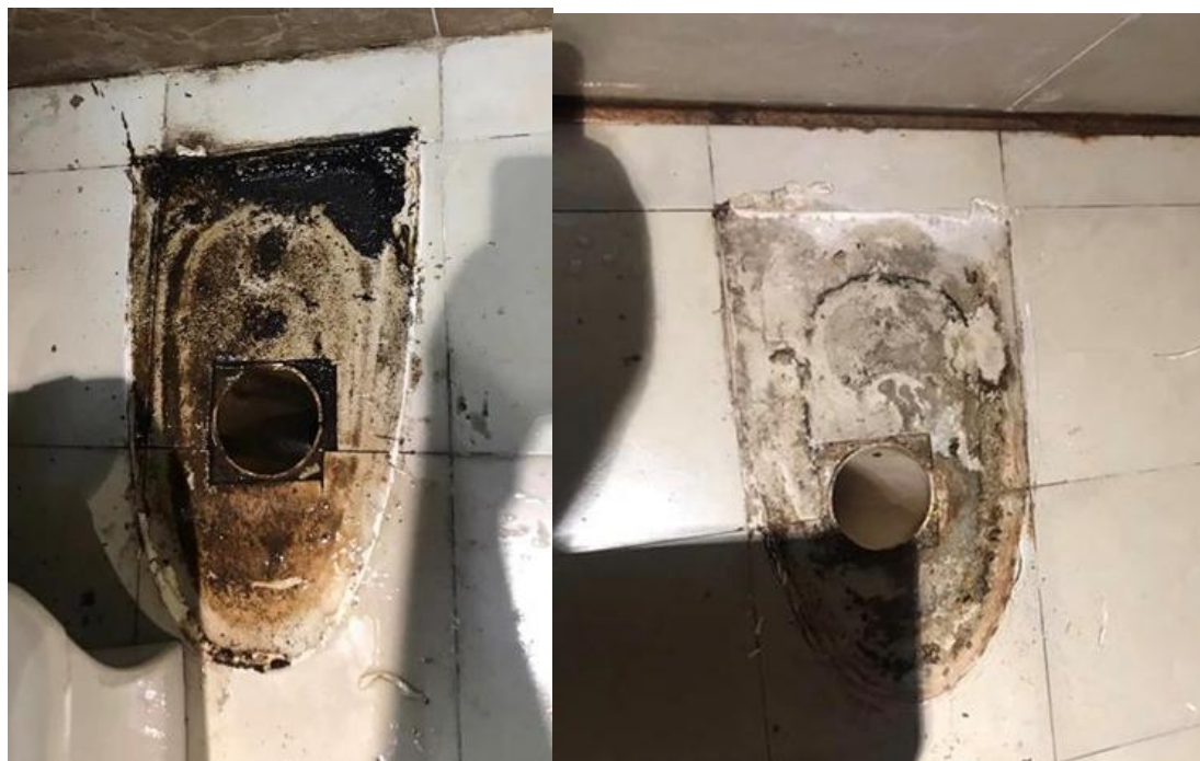
Figure 1. (a) Floor drainpipe under a vertical outlet toilet in remodeled room 8326 showing signs of leakage and poor seal; (b) Improperly installed toilet off the drainpipe center in room 8623 at Dinis Hotel.
