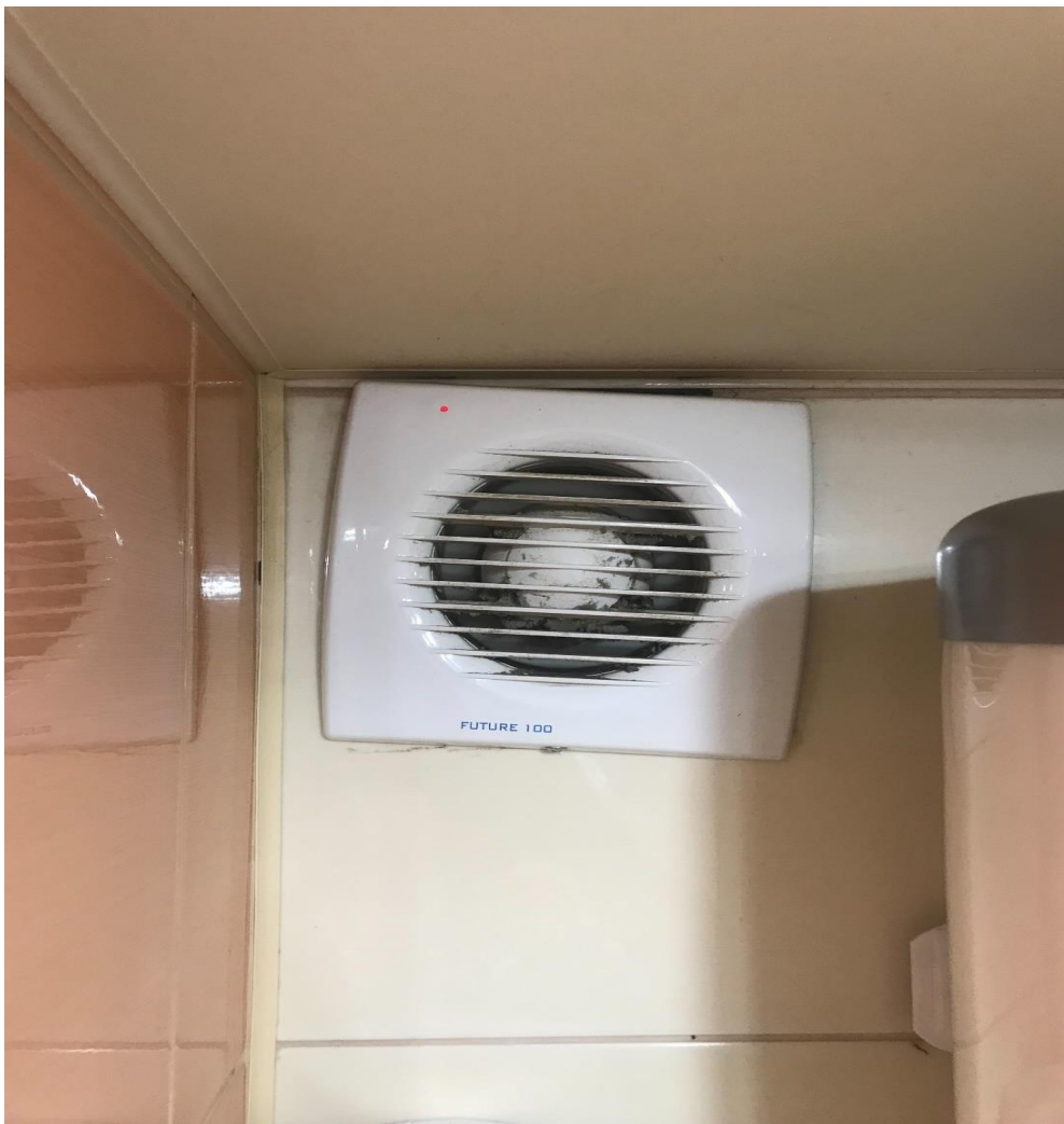
Figure 1. Wall fan installed in the toilet of an apartment on the 3 rd floor of a 9-story building in Tomsk.
