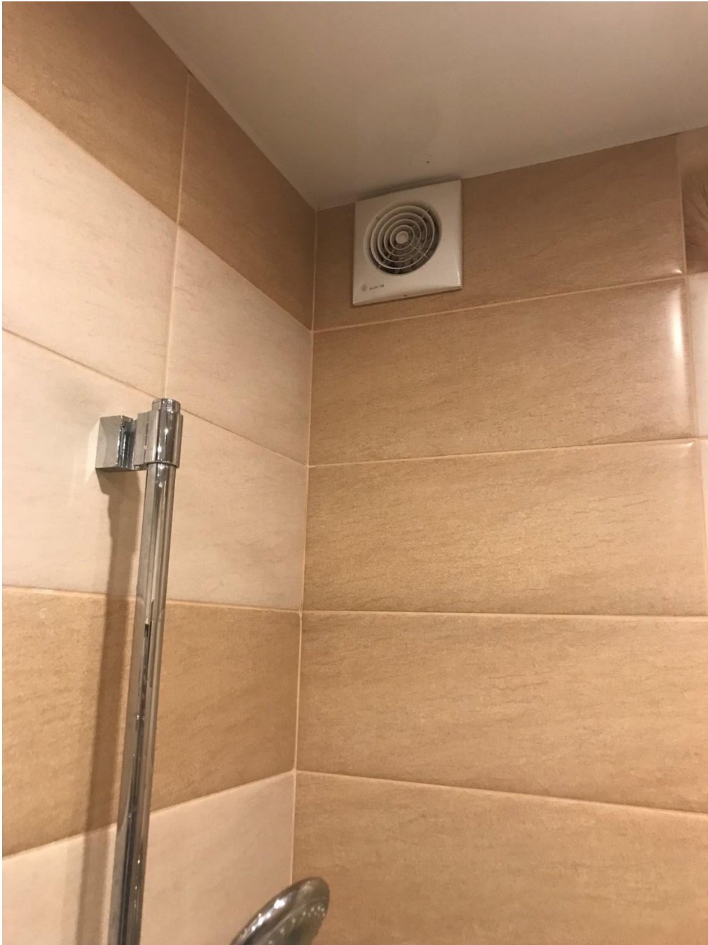
Figure 2. Wall fan installed in the bathroom of an apartment on the 9 th floor of a 10-story building in Tomsk.
