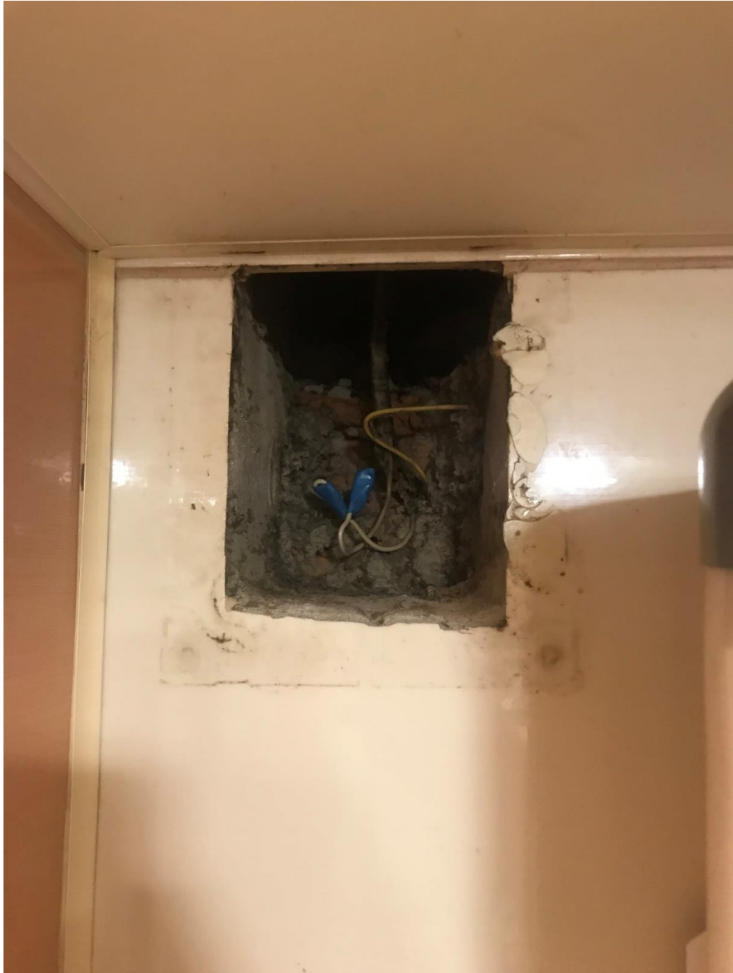
Figure 3. The air vent in the bathroom of a residential apartment in Tomsk without a fan.
